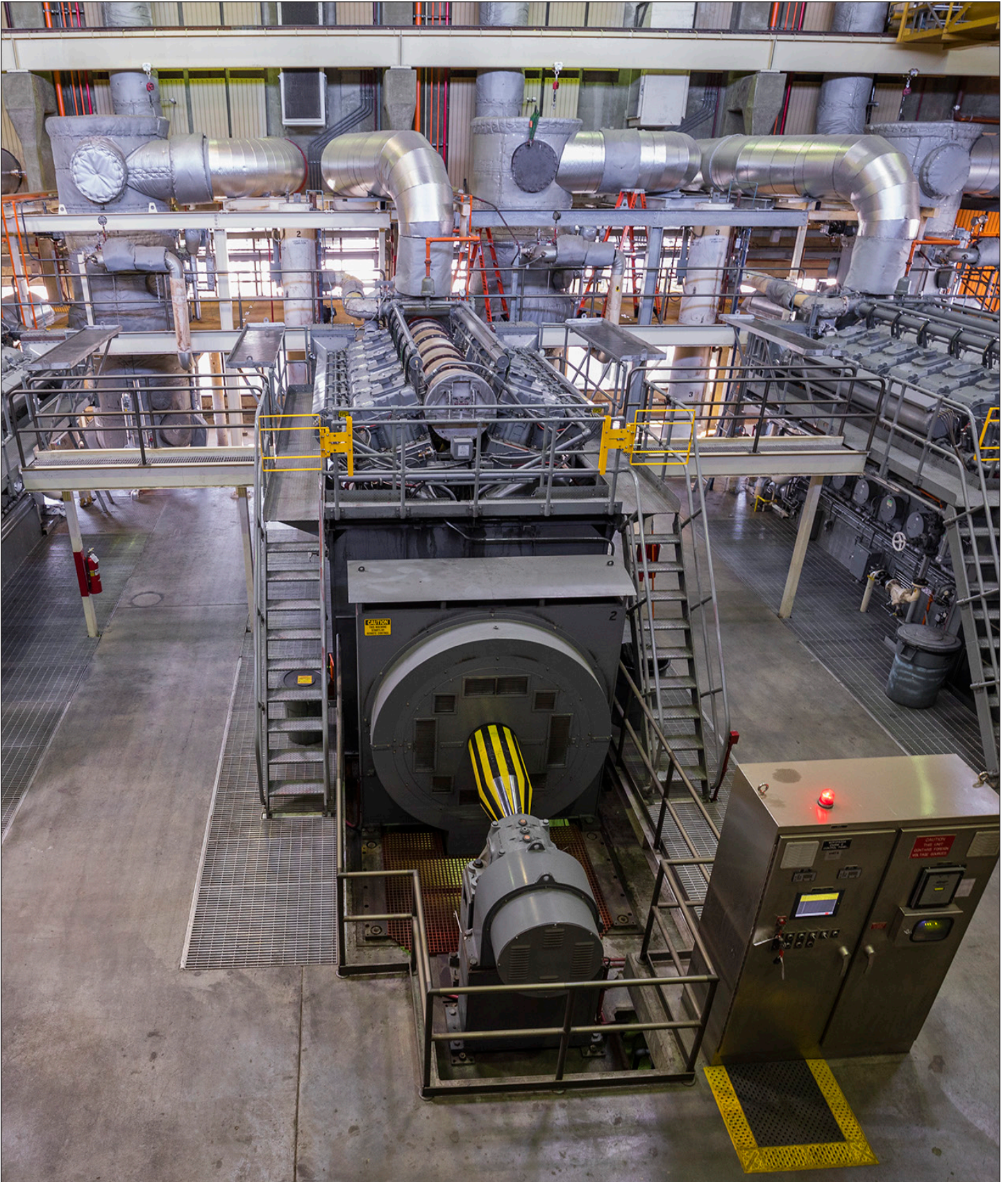
Internal combustion engine at the Central Generation Facility at Plant No. 1 in Fountain Valley.
