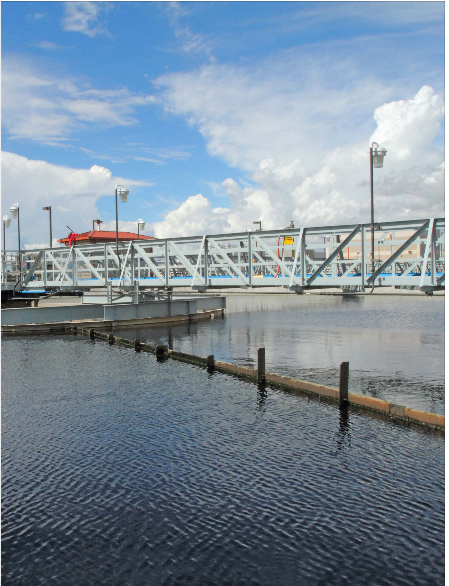
Secondary Clarifier Plant No. 1 in Fountain Valley.
