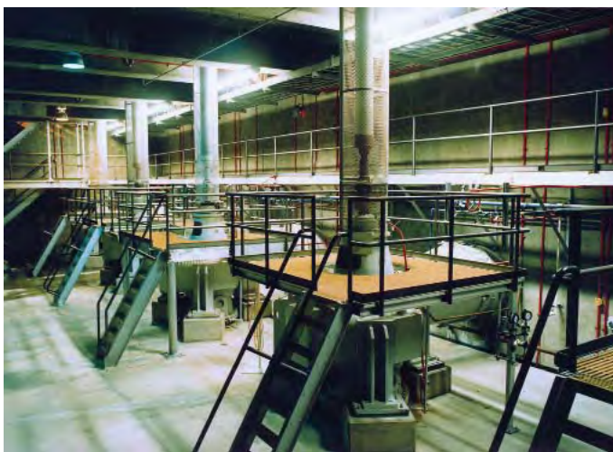
Inside the headworks pump room, bottom of motors.
