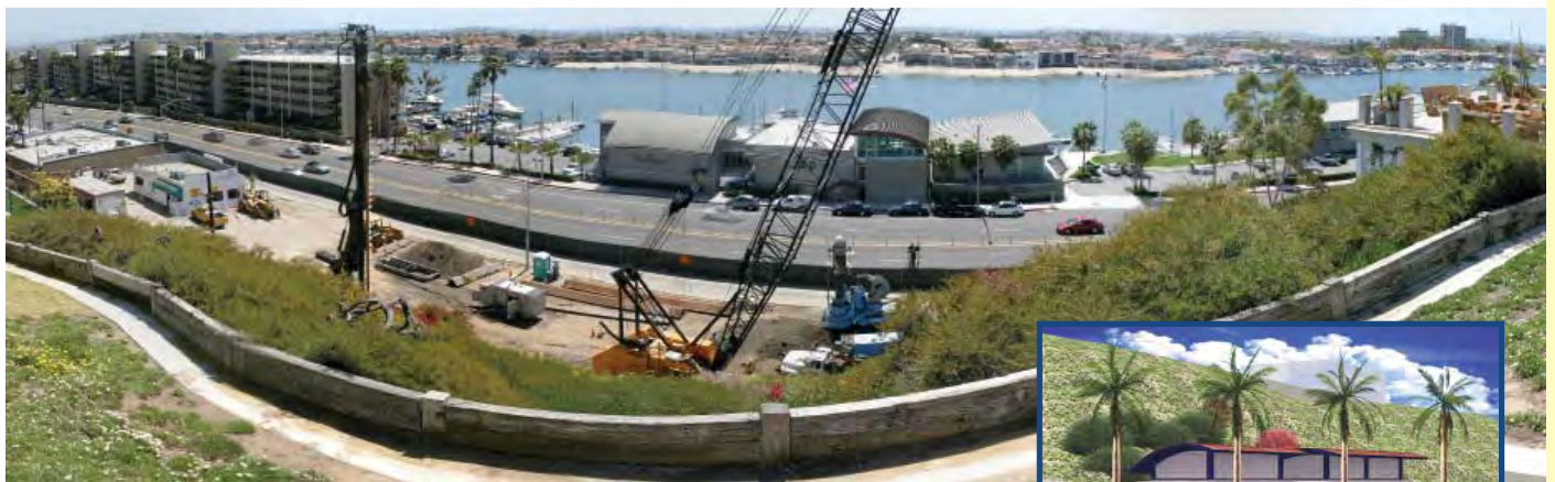
Construction site and artist rendering of the new Rocky Point Pump Station in Newport Beach.
