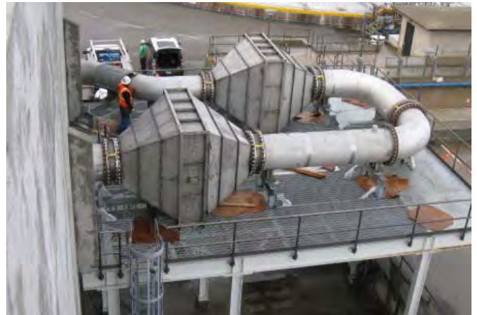
Project No. J-79 – OCSD is pilot testing new technologies to remove air toxics from internal combustion engine exhaust. After the successful testing of catalyst system technology at Plant No. 2, a two-step catalyst unit with a digester gas pre-cleaning system was installed at Plant No. 1 to test its capabilities of reducing NOx and CO emissions. Full-scale installation on eight engines of this new emission control technology is estimated at $31 million.
