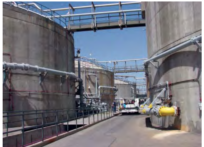
There are a total of 12 sludge digesters at Plant No. 1 that treat an average of 126,000 wet tons of solids a year.
