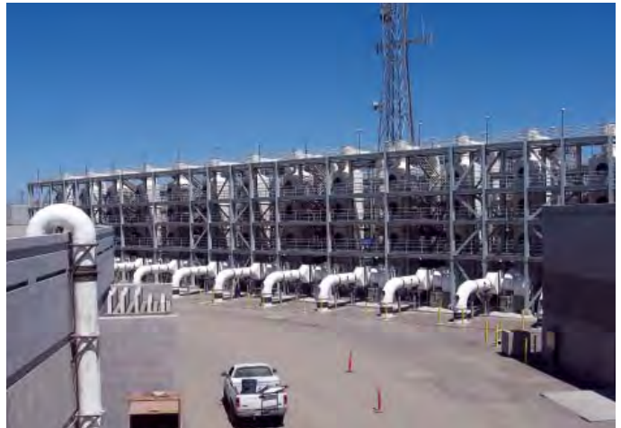
One of the new odor control structures of the headworks improvement project includes a five-story complex that houses 16 biological and eight chemical air scrubbers that remove odors from the foul air piped from various other headworks processes.
