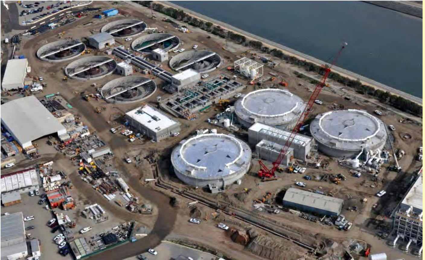
Aerial view of the new trickling filter project construction site at Plant No. 2.
