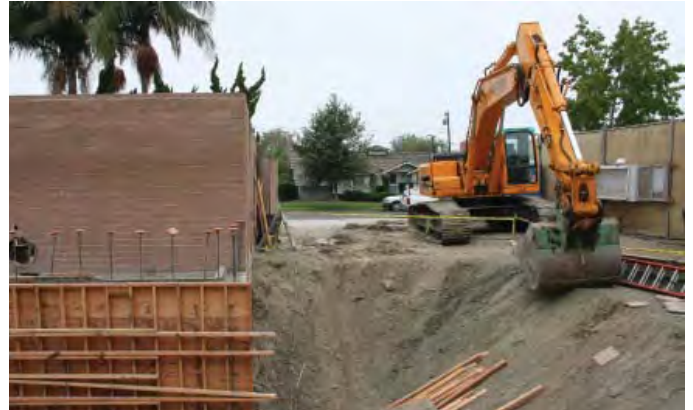
The Westside Pump Station is another challenging site for construction, as the station sits between two houses in a residential community.
