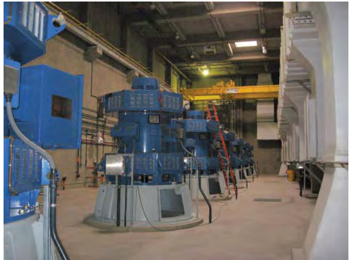
The headworks improvements project replaces the influent pumps with five new 700 hp pumps capable of raising the water almost four stories to allow gravity to push the flow through the rest of the treatment plant.
