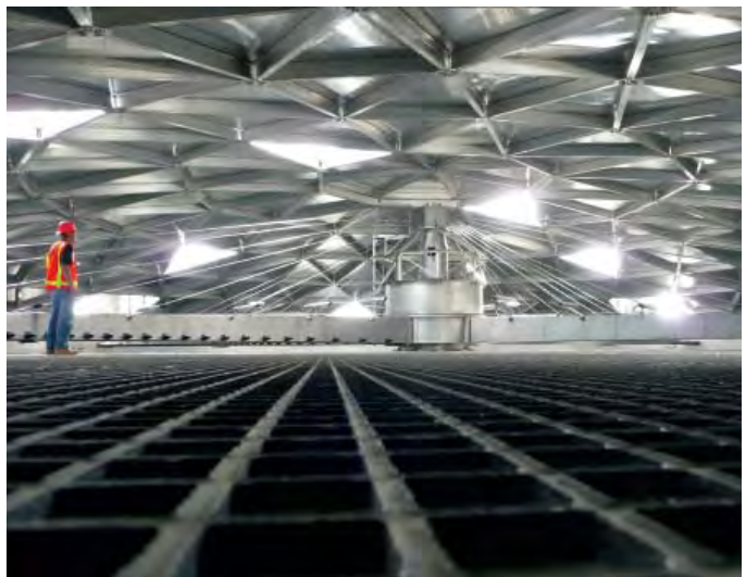
Inside a new dome-covered trickling filter at Plant No. 2. Similar to the trickling filters at Plant No. 1, modules of plastic media fill the 2-story filters. 5.3 million sq. ft. of media surface area (enough to cover the Staples Center six times).
