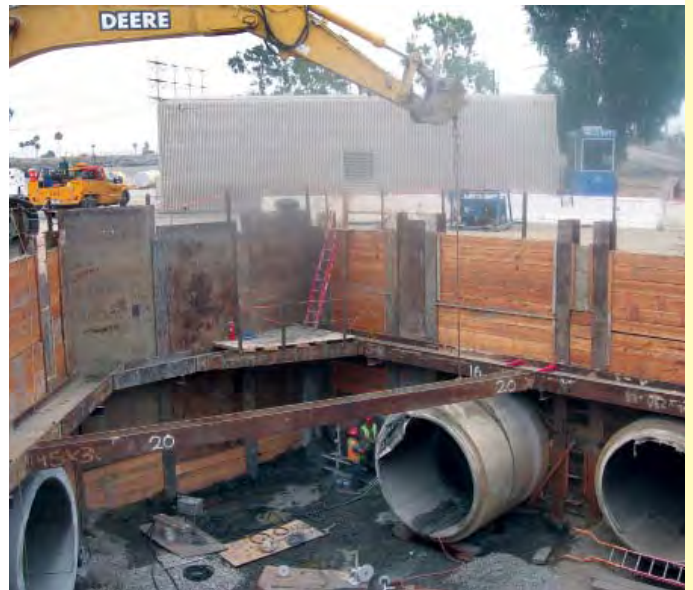
P1-102 construction includes a new secondary effluent junction box. The new junction box will allow the effluent from the new aeration basin facility to combine with effluent from the existing facilities. The pipelines in the photo are two 9-foot diameter plant effluent lines.
