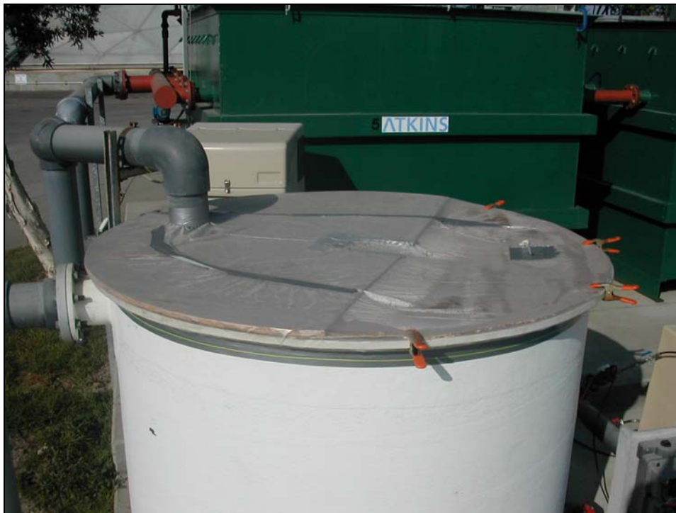
Figure B1 ABR pilot plant at effluent tank covered to assess build-up of methane gas
