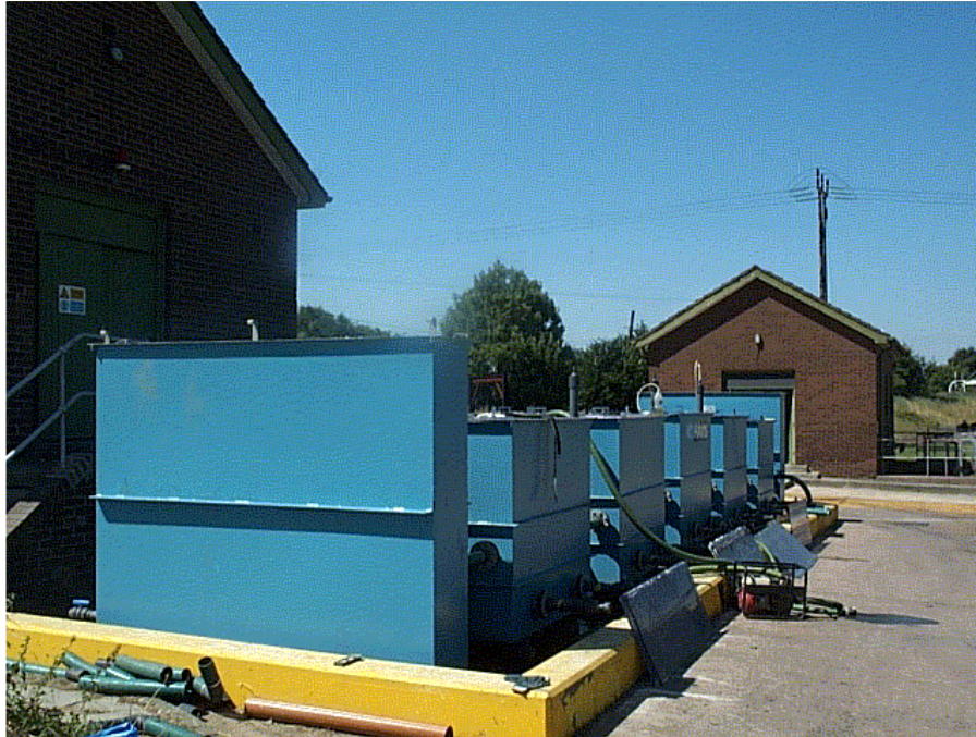
Figure 3.1 ABR pilot plant at Ellesmere Port
