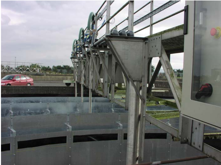
Figure 3.4 Gantry showing the de-sludging lines
