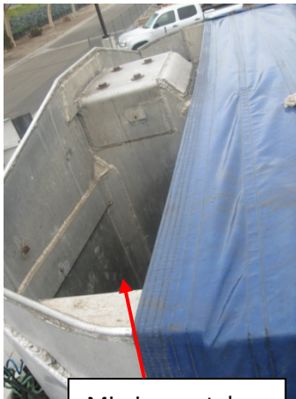
Missing metal splashguard.
